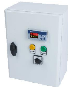
Fig. 48 - Continuous controller in the control cabinet
